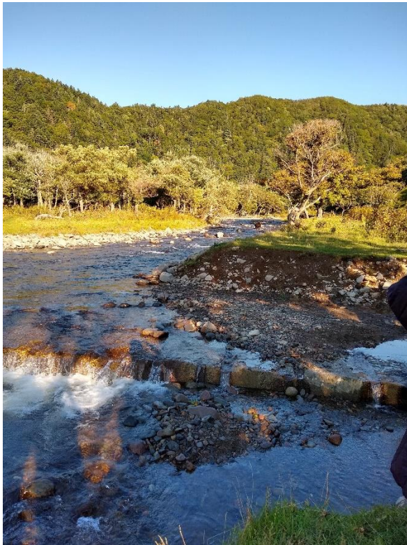
Figure 1. Image of Rurua River Dam #3 following initial phase of concrete removal (foreground). Some of the upstream riparian trees that are perceived to be at risk are evident in the upper part of the image. A brown bear appearing in the upstream reach was also observed foraging during the visit (©IUCN/Peter Rand).
